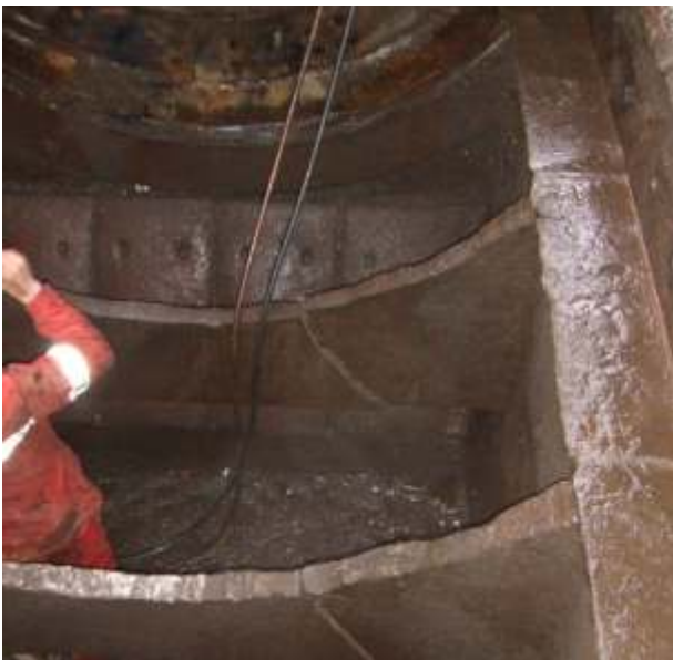
Before the repair
